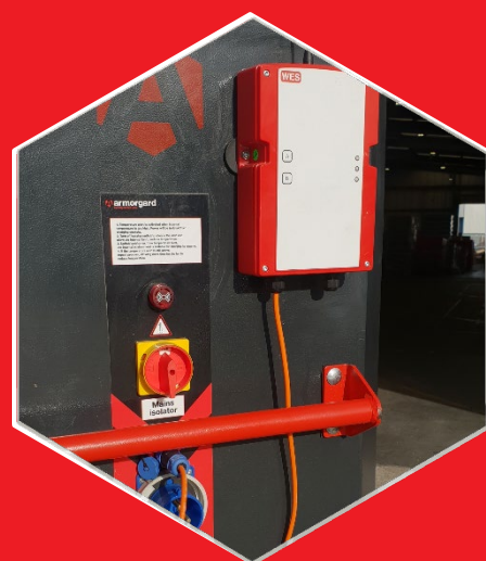
Multiple alert systems: fire alarm system & GSM alerts
