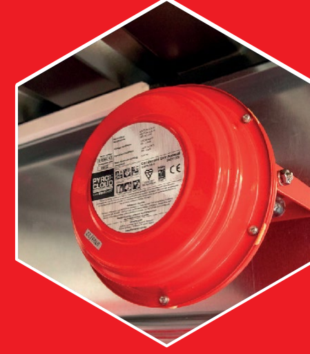
Fire suppression and alert systems should still operate without mains power
