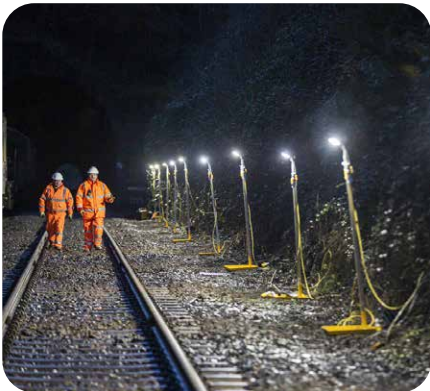
Pro-Link's in use on side of track, 10m spacing
